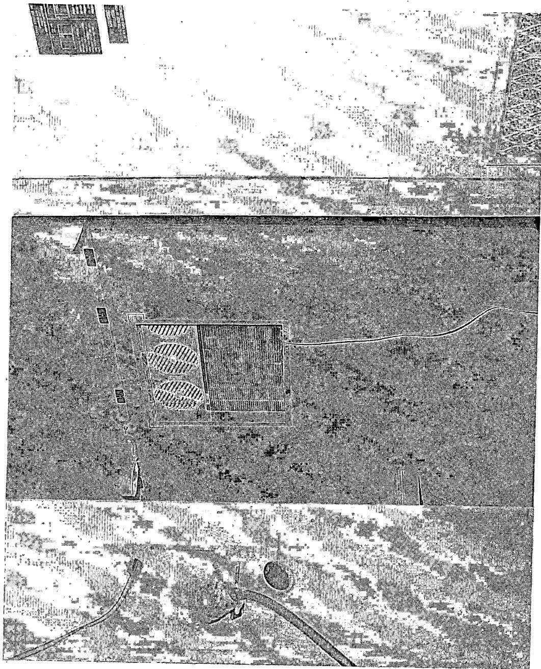
Figure 34 - Interior of Hut Showing Air Conditioner
