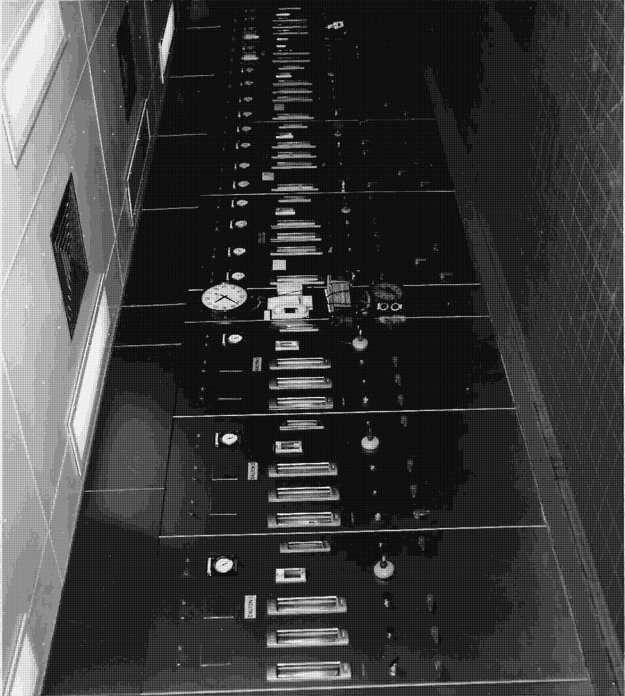
ELECTRONIC MONITORING/CONTROL SYSTEM
