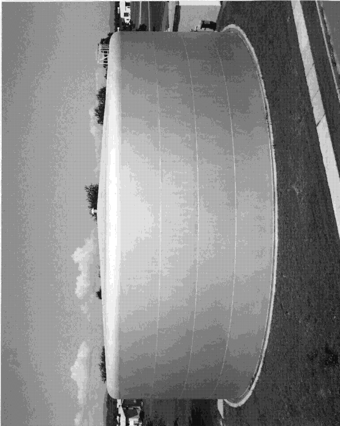
P-3100, WATER STORAGE TANK (2,000,000 gallon capacity)
